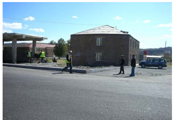
Renovated building of Bagrevan village Mayor and rehabilitated road. Civil works still in progress.
